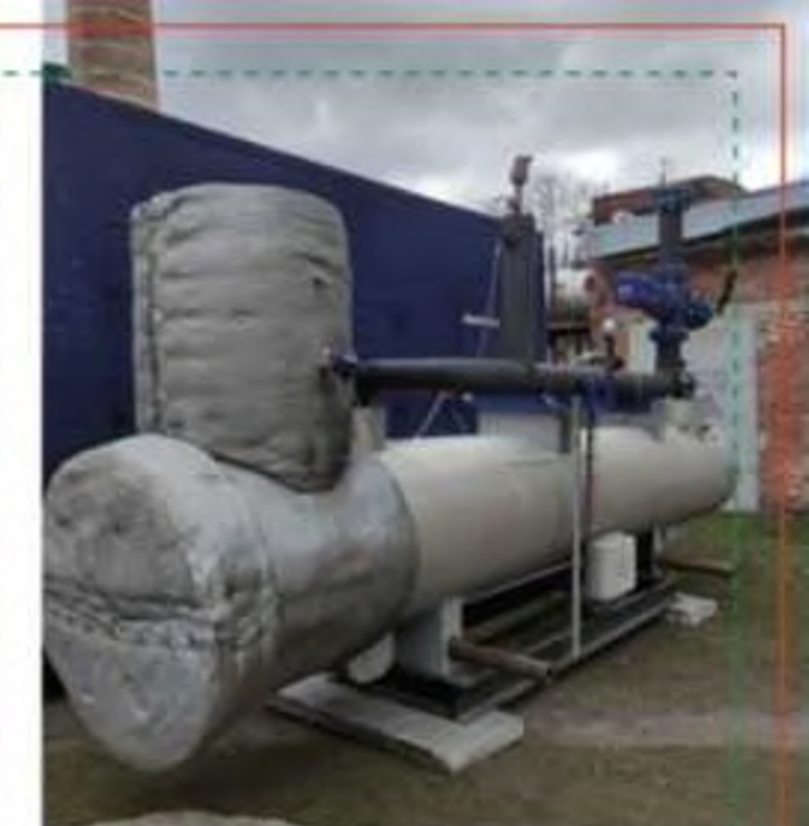
Photo of the cogeneration unit
